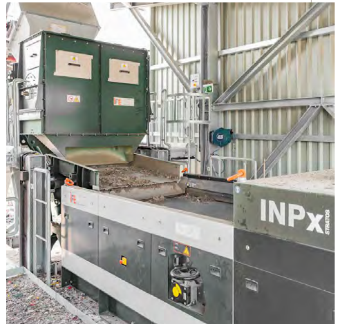
Wirbelstromscheider in Recyclinganlage Eddy current separator in a recycling plant
